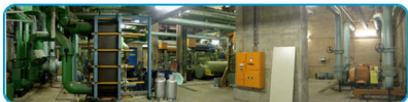
Plant room in Level 1
