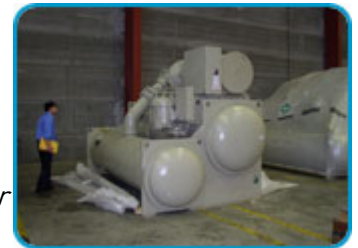
New McQuay Chillers in Warehouse
